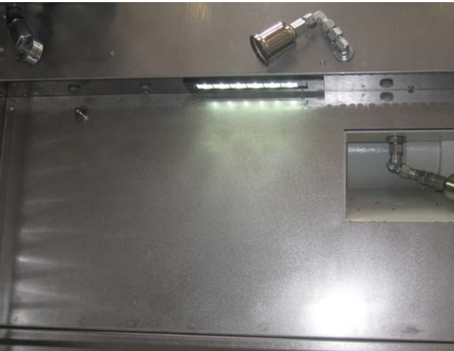
Figure 11 Extinguishing nozzle and heat detector/temperature sensor in the interior of the machine
